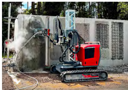
Aquajet showed its fleet of equipment and performed hydrodemolition demonstrations at the company's 2024 World Tour event in Germany.
