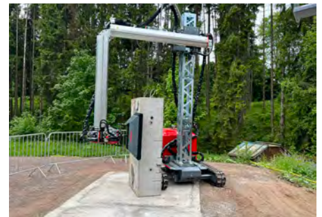
Attendees at Aquajet's World Tour in Germany saw a variety of Hydrodemolition demonstrations with state-of-the-art equipment.
