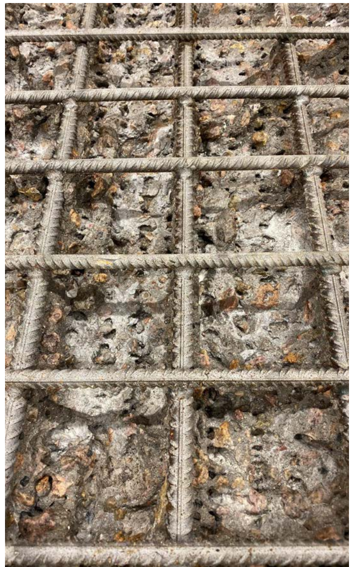
Example of surface with pipeholes that appears in lines.
